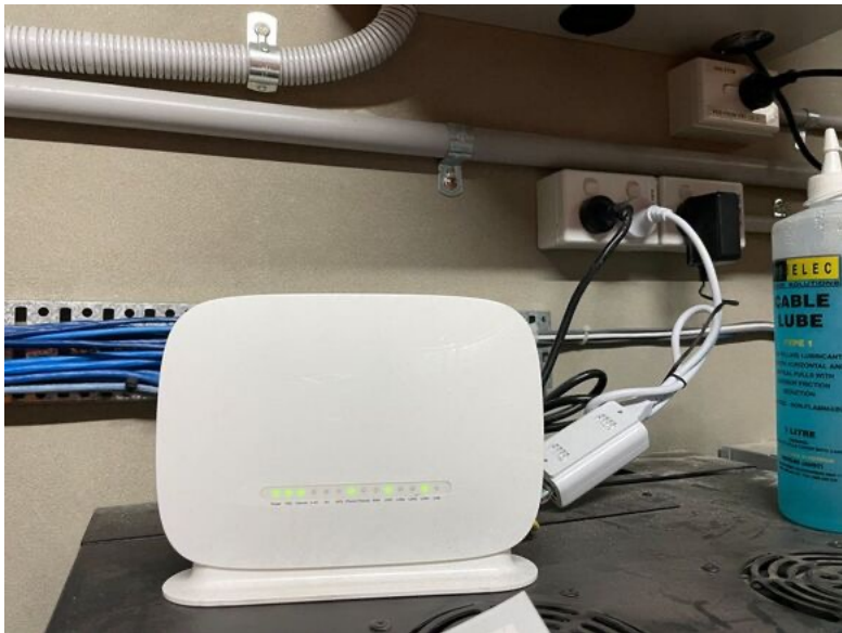
Wi-Fi router in main switchroom
