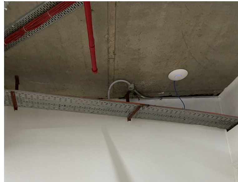
Wi-Fi repeater on roof of basement carpark
